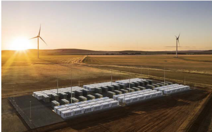
The Tesla big battery has responded rapidly to system outages.
