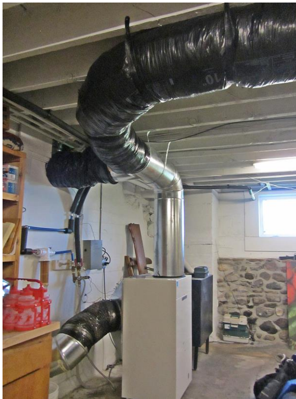
Self-Ducted to Living Area
