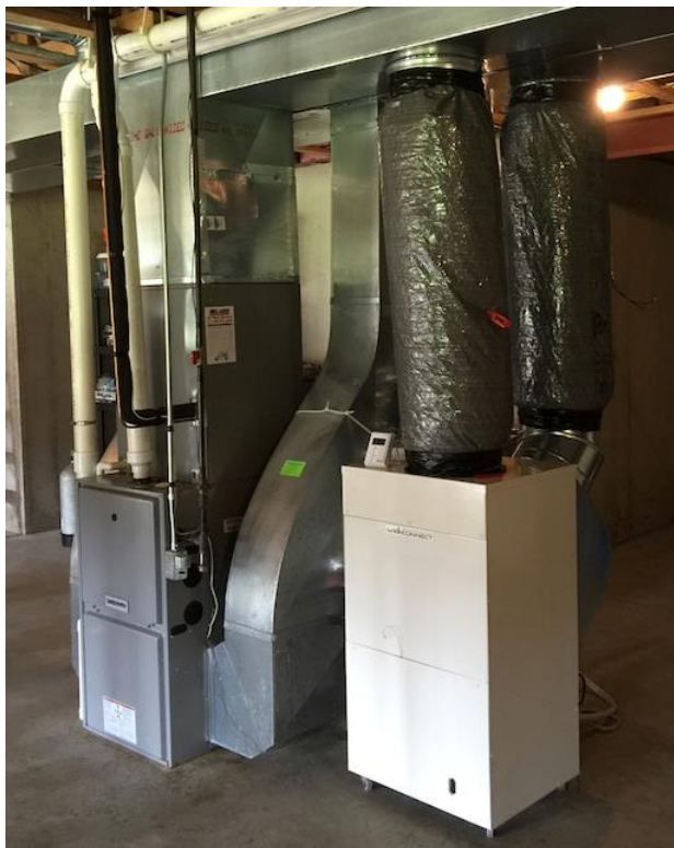
Integrated with Existing Furnace
