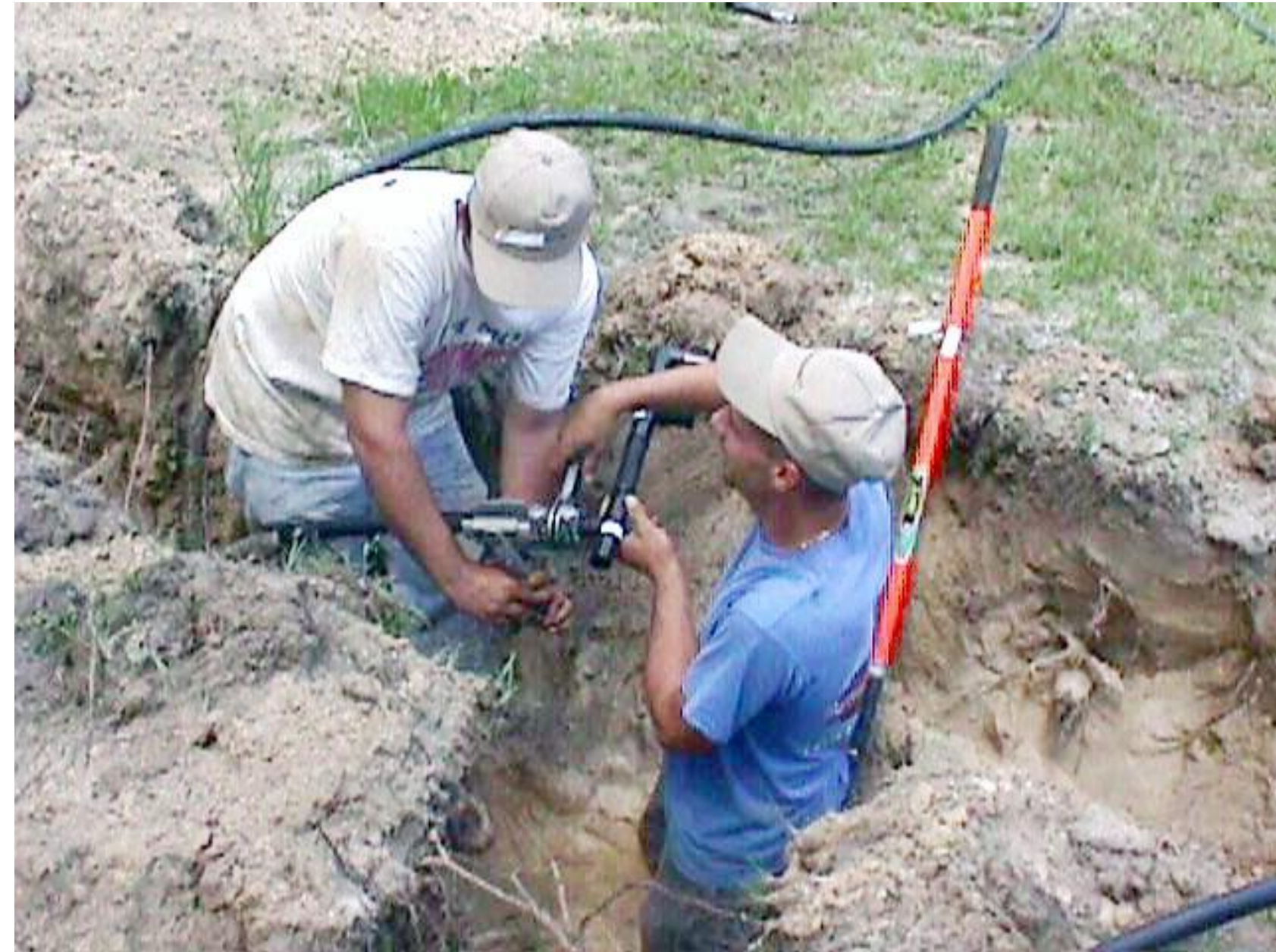
Installing GHP pipes for residential housing in South Carolina. Photo by Belton Tisdale. NREL pix 12372
